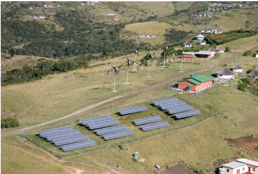
Figure 3 Hybrid mini-grid system at Lucingweni village
