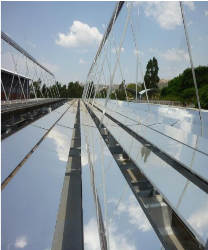
Figure 8 Solar thermal cooling at MTN headquarters, Johannesburg (photo: D. Holm)
