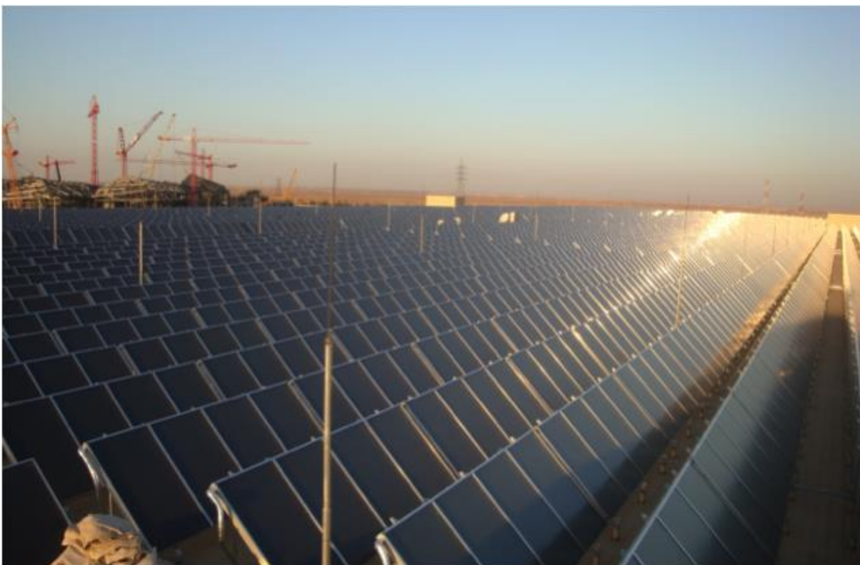
Figure 5 Biggest installation worldwide in Saudi Arabia 36 000m 2 or 25MWth (photo: AEE-Intec)
