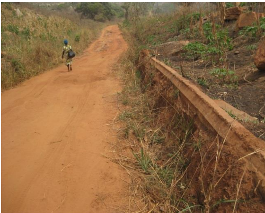
Figure 2: Poor Kerb Drainage Structures Leading to Severe Erosion
