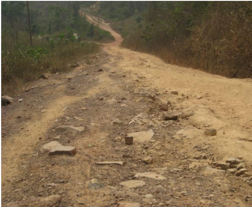
Figure 1: Lack of Roadside Drains Leading to Severe Sheet Erosion
