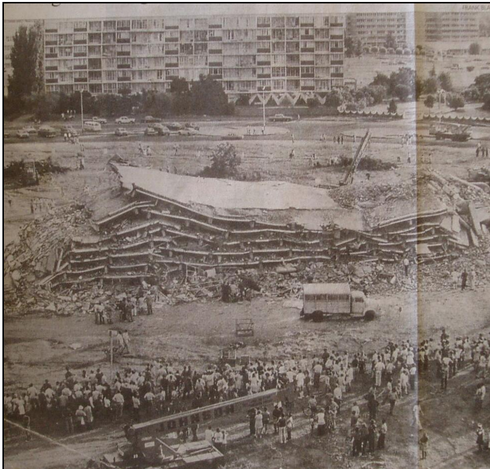
Figure 2. Damage to an apartment block in Welkom caused by a M_L=5.2 tremor on 8 December 1976
