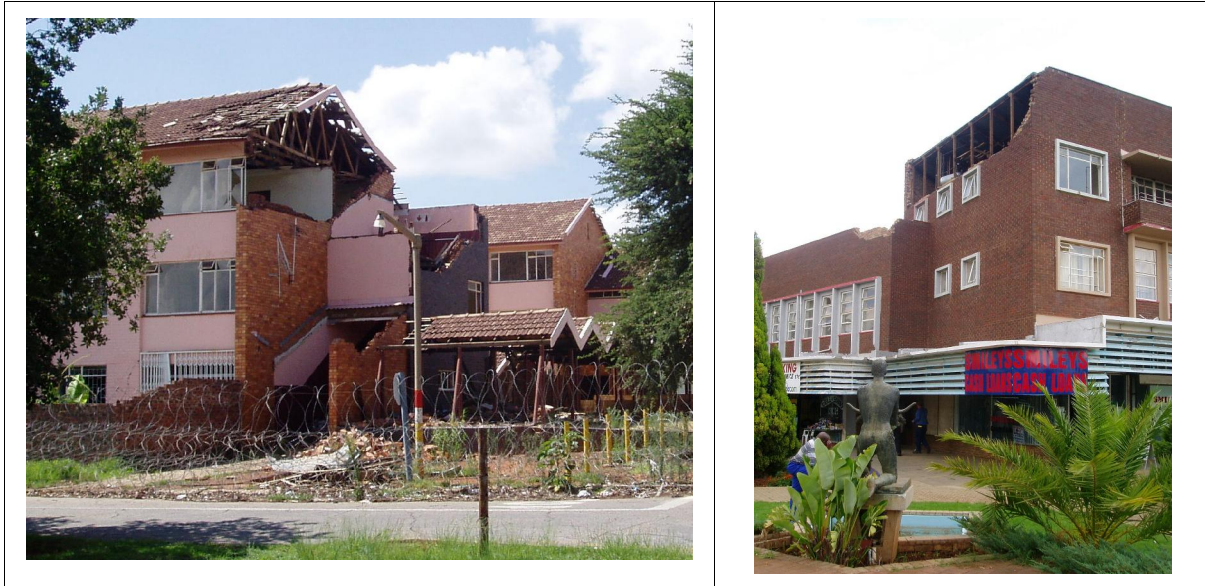
Figure 1. Damage in Stilfontein caused by the M_L=5.3 tremor on 9 March 2005
