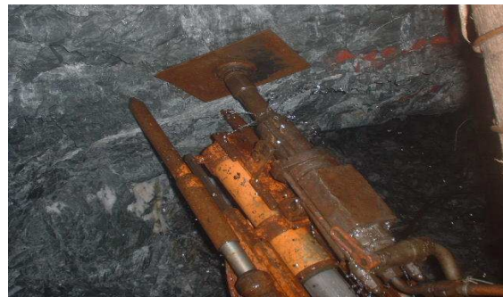
Figure 8. Spin-to-stall installation of a roofbolt in the hangingwall close to the stope face.
