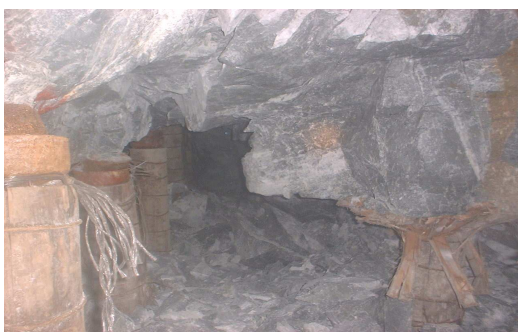
Figure 7. Seismically induced fall of ground at the top of the panel face area
