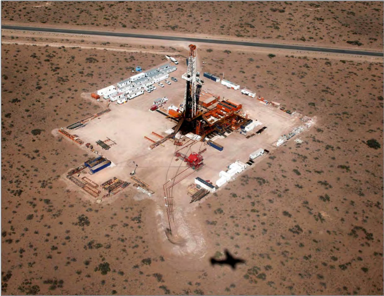
Figure SPM 1.5: Wellpad layout with a drill rig of about 40 m in height within an arid environment in Argentina. (Source:REUTERS, http://www.vcpost.com/articles/5923/20120925/sidewinder-drilling-to-buy-union-drilling-for-139-mln.htm ).
