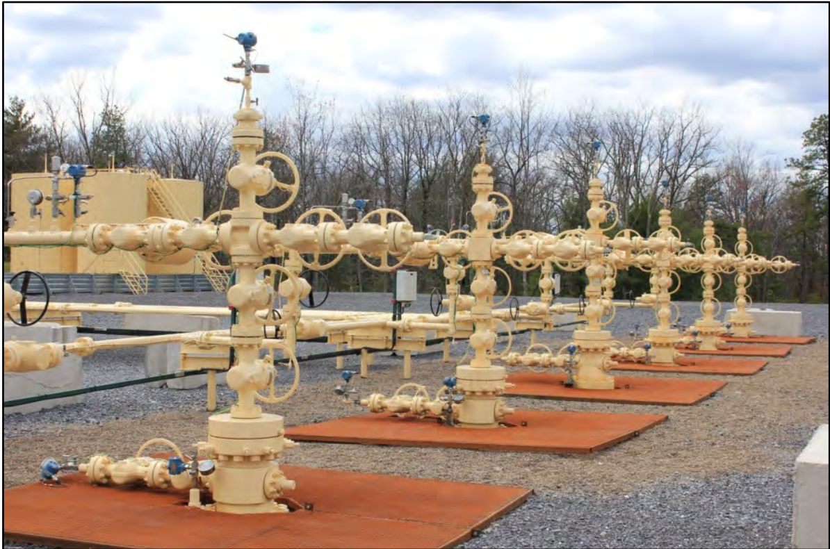
Figure 1.37: Cluster of producing wellheads (Source: Tom Murphy (n.d.), Pennsylvania State University, USA)
