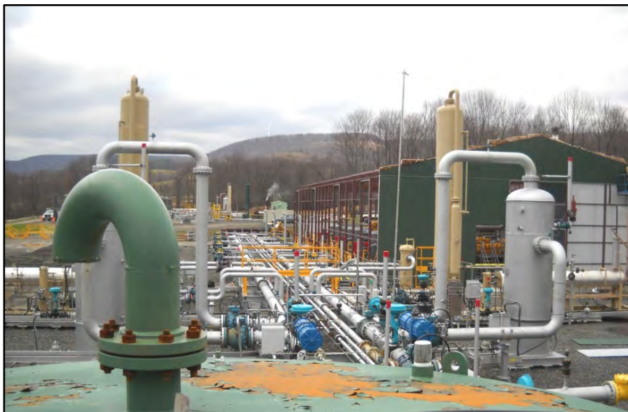
Figure 1.39: Example of a centralised gas compressor station. Compressed gas would be exported from this facility, via pipeline, to a downstream facility such as a CCGT power station (Source: Tom Murphy (n.d.), Pennsylvania State University, USA).
