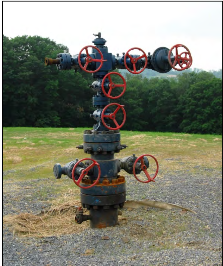
Figure 1.34: Surface equipment in place for a suspended well (Source: Tom Murphy (n.d.), Pennsylvania State University, USA)
