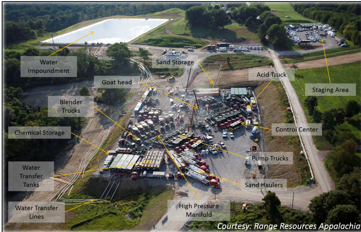
Figure 1.29: Example of a fracking process underway in Appalachia, with the main equipment and facilities involved indicated (Source: Range Resources Corporation).
