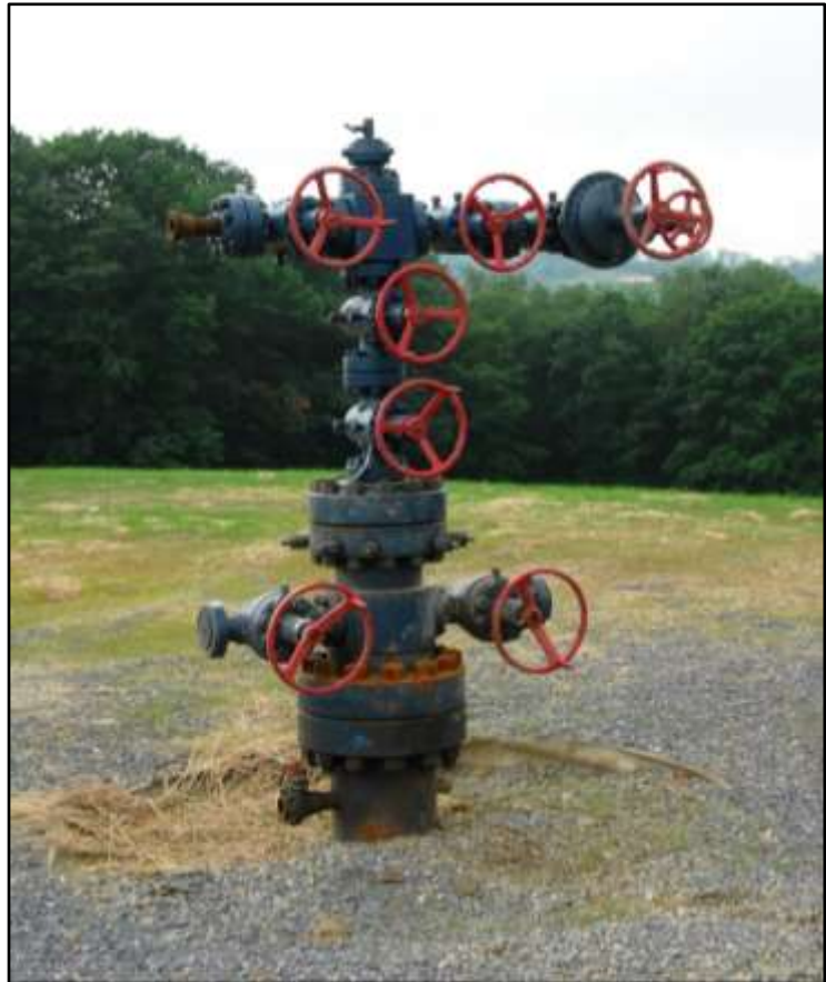
Figure 1.34: Surface equipment in place for a suspended well (Source: Tom Murphy (n.d.), Pennsylvania State University, USA)
