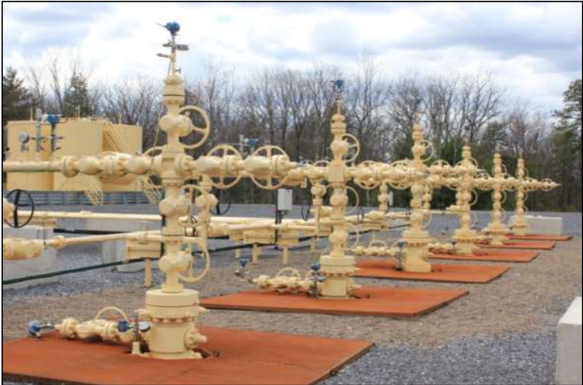
Figure 1.37: Cluster of producing wellheads (Source: Tom Murphy (n.d.), Pennsylvania State University, USA)
