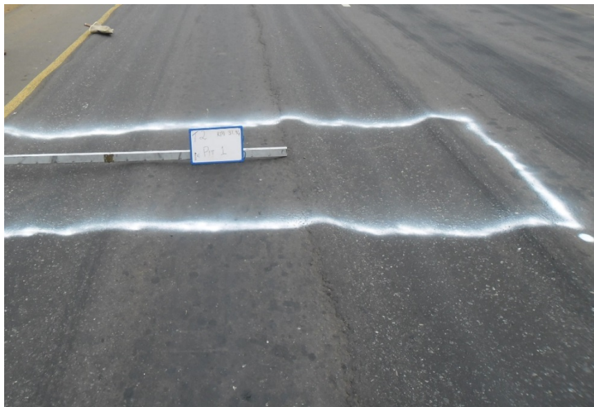
Figure 2: Extent of rutting on Project B
