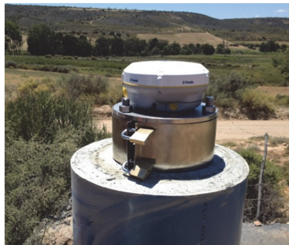
Figure 4. Receiver installed on stainless steel mount at Z031 with security band installed.
