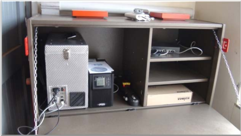
Photo 5-2: The silver box is where the server was placed in a secure, folding container which had to be placed in a secure and ventilated area in the school.
