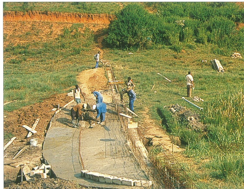
Community water supply scheme
