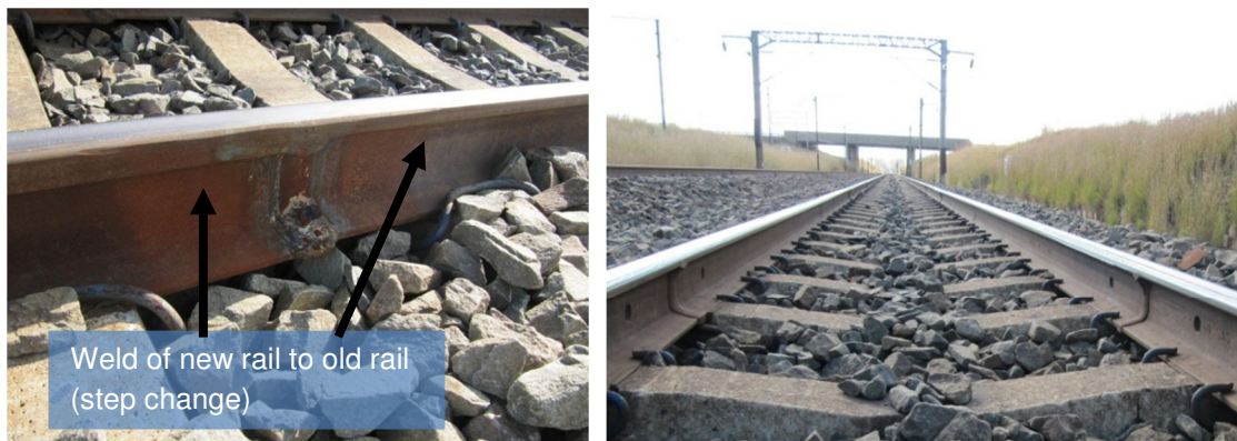
Figure 9 New rail welded to old rail and frequency welds in old rail.
