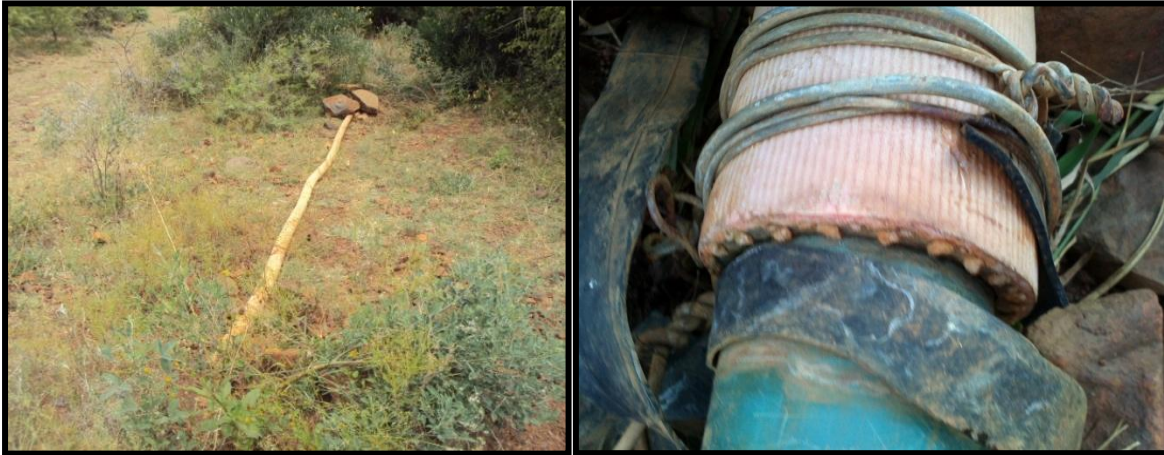
Figure 3: Mountain water pipe exposed above ground (left) and poor pipe joint (right)
