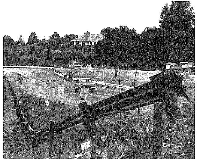
Failure of the Rickivy embankment near Pietermaritzburg
