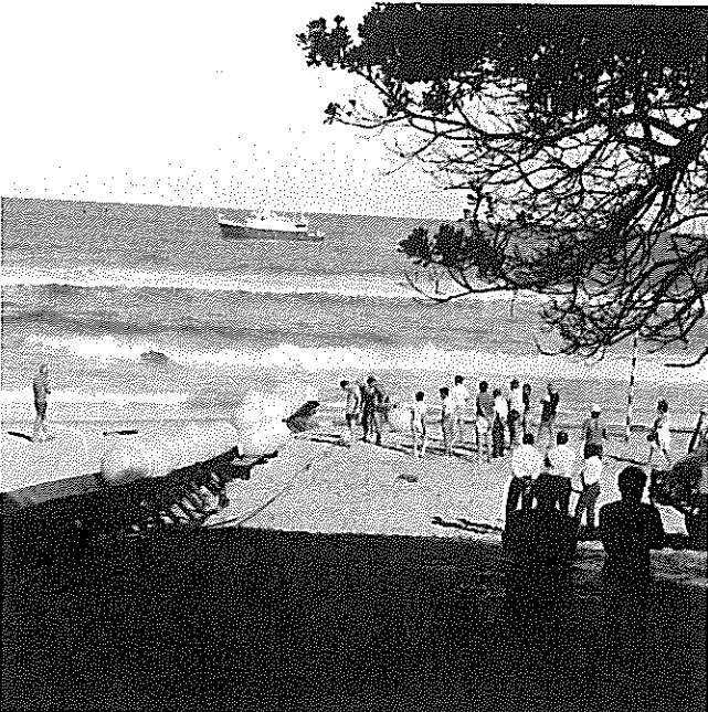
A cable for an electric shark barrier being laid in the sea off the Natal coast.
