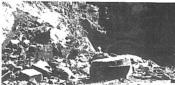
The Geomechanics Division undertook an analysis of the stability of the entrance to this tunnel to establish whether further collapses might occur.
