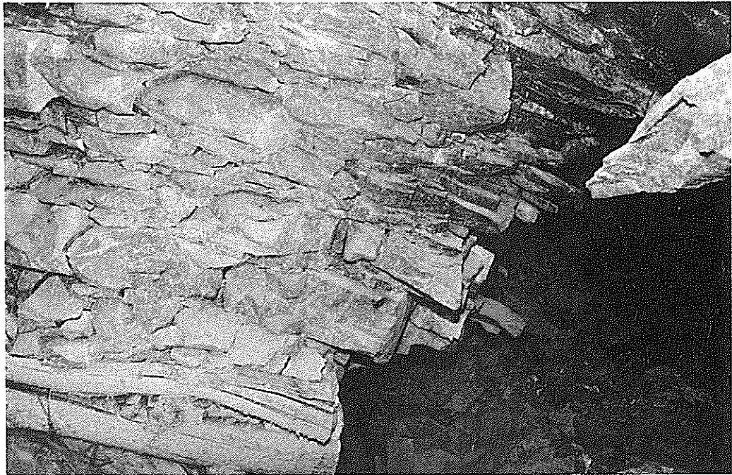
Figure 6 A VIEW SHOWING THE INCIDENCE OF HANGINGWALL-PARALLEL FRACTURING IN THE FAIL ILLUSTRATED IN FIGURE 5
