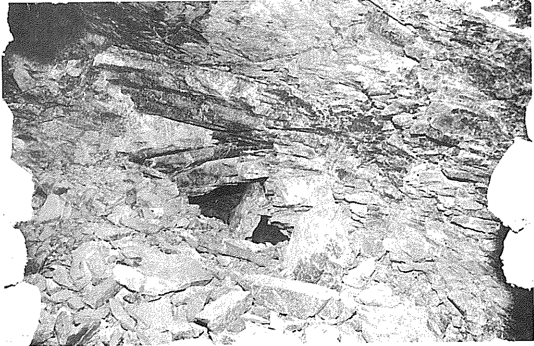
Figure 5 PART OF A MAJOR FAIL DUE TO A ROCKBURST AFFECTING THE HANGINGWALL OF THE 1024 - 58 W1 GULLY ON WESTERN DEEP LEVELS
