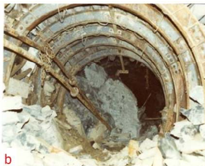
(b) Damage in tunnel at 2 000 m below surface following M_L=4.2 event at West Driefontein Gold Mine, 1983.
