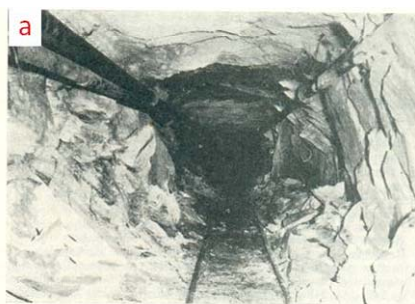
(a) Slabbing of tunnel sidewall at 9 000 ft (2 743 m) below surface at Robinson Deep Mine, 1957 (Leeman, 1959).
