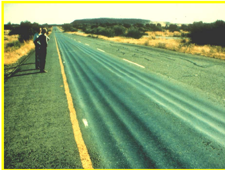
FIG. 2. Plastic deformation (or rutting/shoving) within the thin asphalt surfacing layer. Note the six lanes of rutting (left and right sides) owing to tire loading combined with poor asphalt mix.
