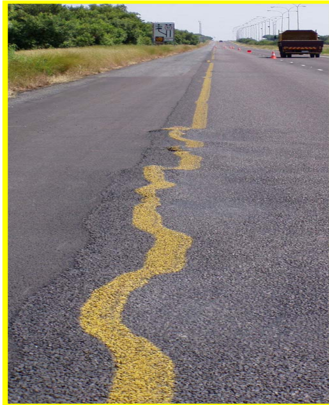
FIG. 9. “Wiggling yellow line” owing to shear failure in a substandard (or wet) granular base layer.
