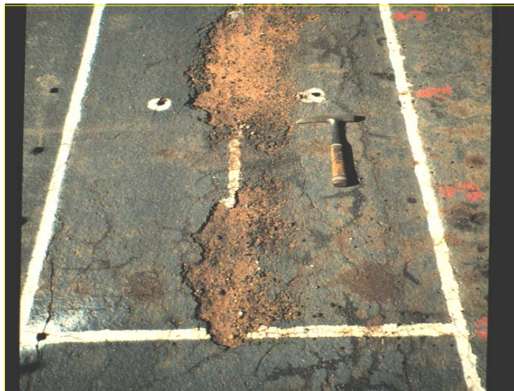
FIG. 6. Surface disintegration in the asphalt surface seal of a low-volume road.
