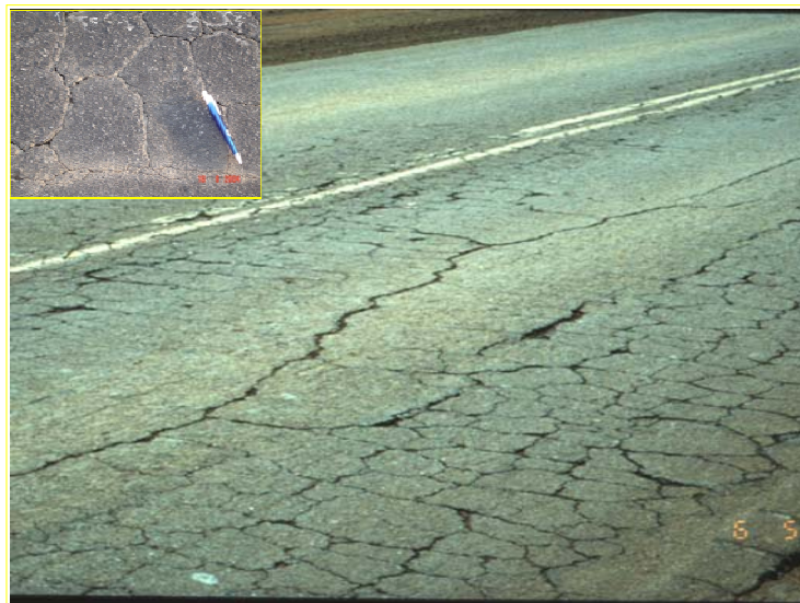
FIG. 4. Fatigue (alligator) cracking of a old and brittle thin surface seal. Note fatigue cracking with some signs of white coloring (pumping of fines) in insert.
