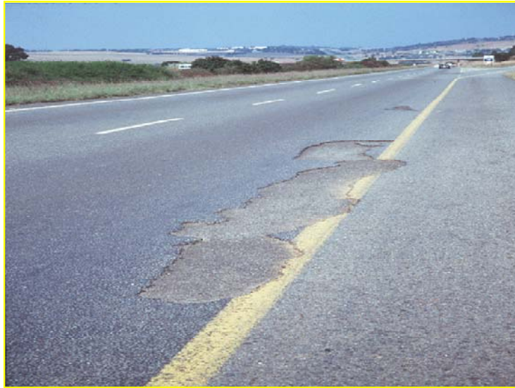
FIG. 5. Delamination of the asphalt surfacing layer from the lower layer.
