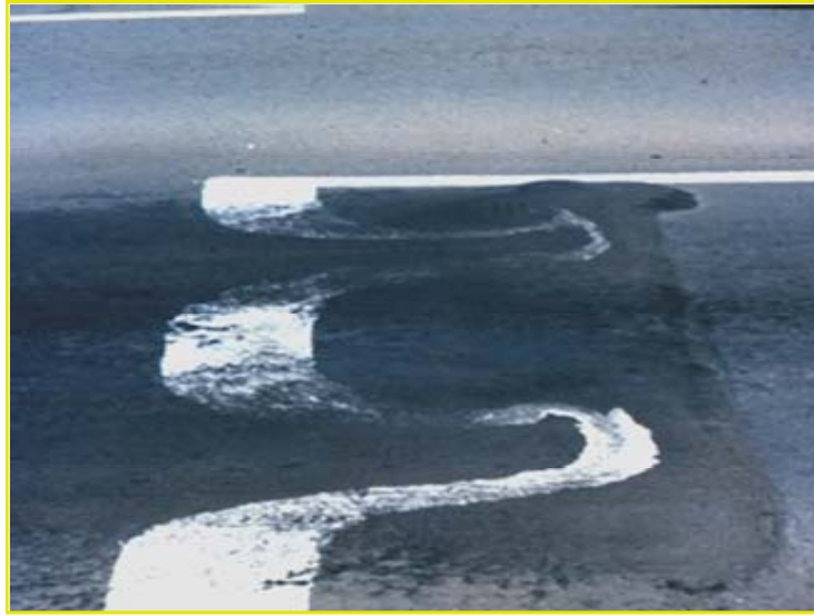
FIG. 3. Horizontal plastic deformation (or rutting/shoving) within the thin asphalt surfacing layer at an intersection. Note the planar backwards deformation depicted by the white lane marking owing to the tractive acceleration forces of tires towards the right of the picture.
