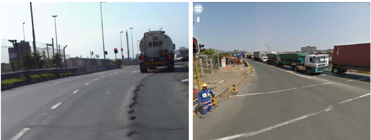
(a) Severe deformation under continuous heavy traffic (b) Traffic situation at the intersection
