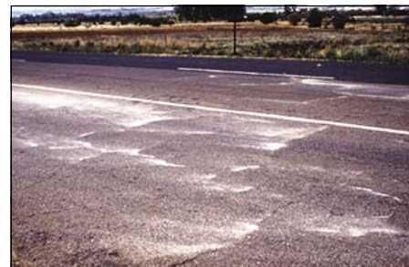
Photo 1 Pumping loose material from a cemented base/subbase pavement at Hornsnek, West of Pretoria during 1985
