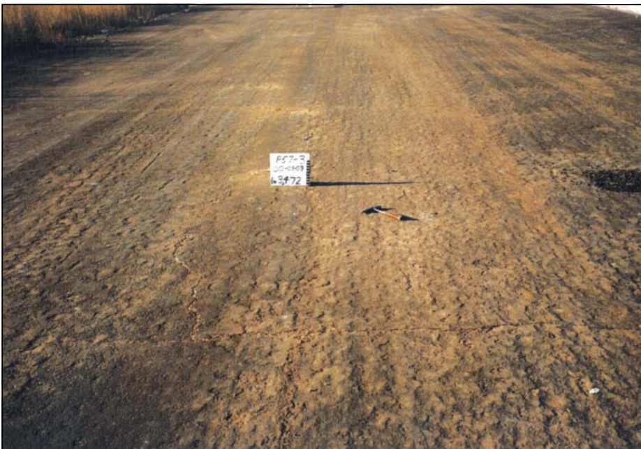
Photo 14 Uneven surface due to use of grid and padfoot rollers too high in base: in addition to undesirable roughness, grid mounds tend to be sheared, and peel and padfoot marks lead to poor bonding and tend to reflect through seal
