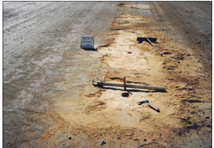
Photo 5 General view of primed, 3% cement-stabilised, weathered granite base after loose to weak upper 25 mm of carbonated material had been hand-broomed off
