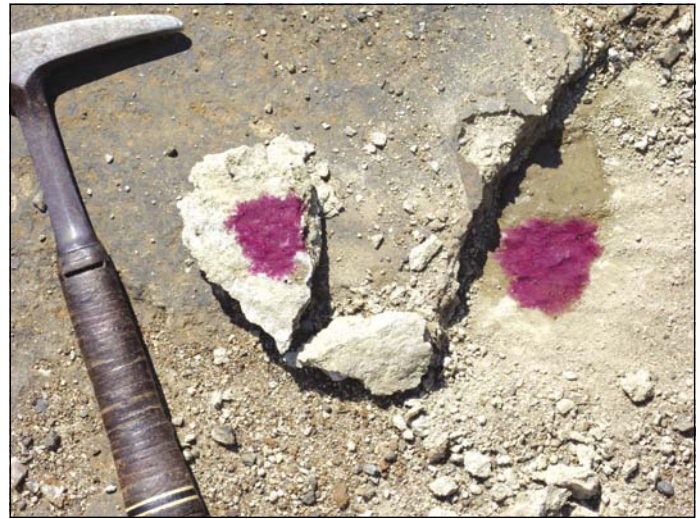
Photo 9 Phenolphthalein tests on a lamination (~ 30 mm) in a recycled cementitious base layer. Most probably the cause of failure in Photo 6. No signs of deleterious carbonation (courtesy of Dr P Paige-Green)
