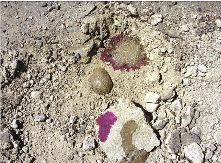
Photo 10 Upper base pavement layer (from Photo 2) showing signs of crushing breakdown and deterioration in the top 30 to 50 mm, with and without signs of deleterious carbonation (courtesy of Dr P Paige-Green)
