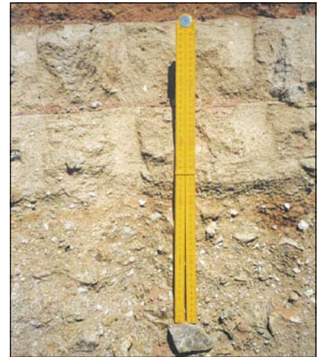
Photo 13 Road layerworks on an excavation. Note some interlayers between 2 nd and 3 rd layers, as well as between 3 rd and 4 th layers
