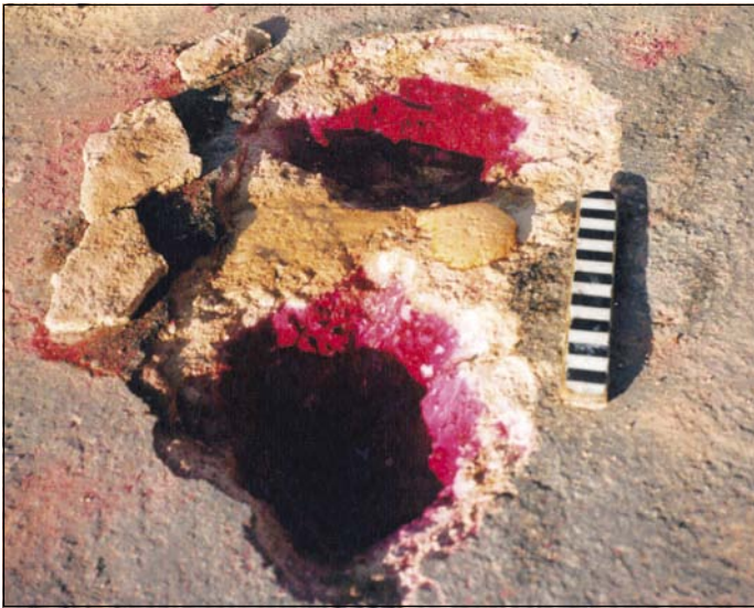
Photo 8 A 7 mm thick "biscuit" on compaction plane, and carbonated and weaker to 15 mm below top of primed, 3% cement-stabilised, weathered granite. Detected by chain drag
