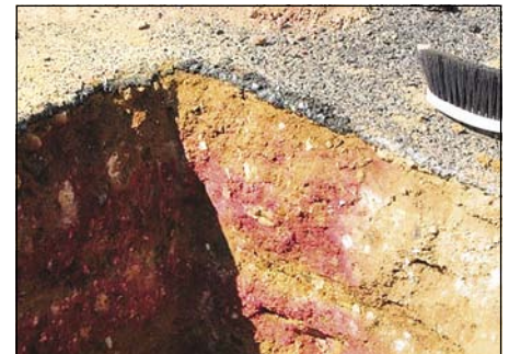
Photo 15 Signs of deleterious carbonation in a cementitious base and subbase pavement (non-pink areas to the right of test pit) (courtesy of Dr P Paige-Green)
