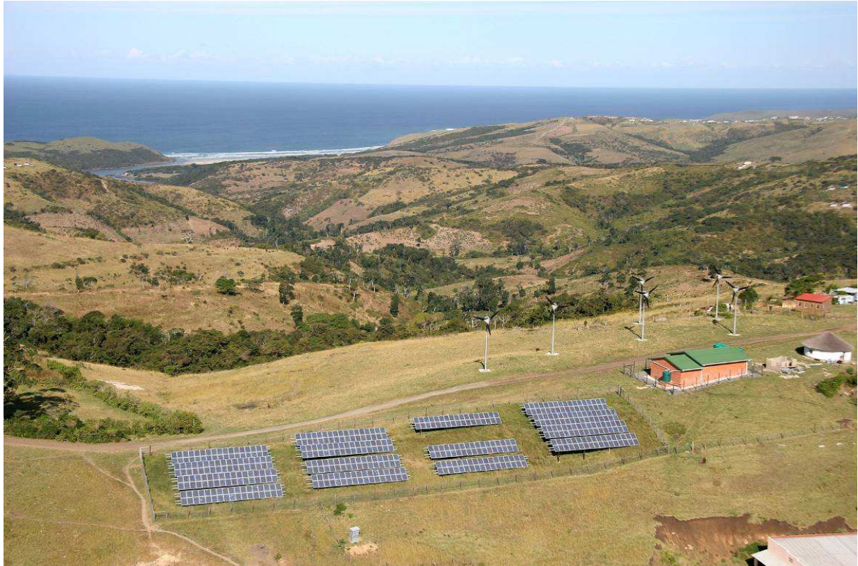
Figure 8: View of Lucingweni 86 kW hybrid mini-grid energy system
