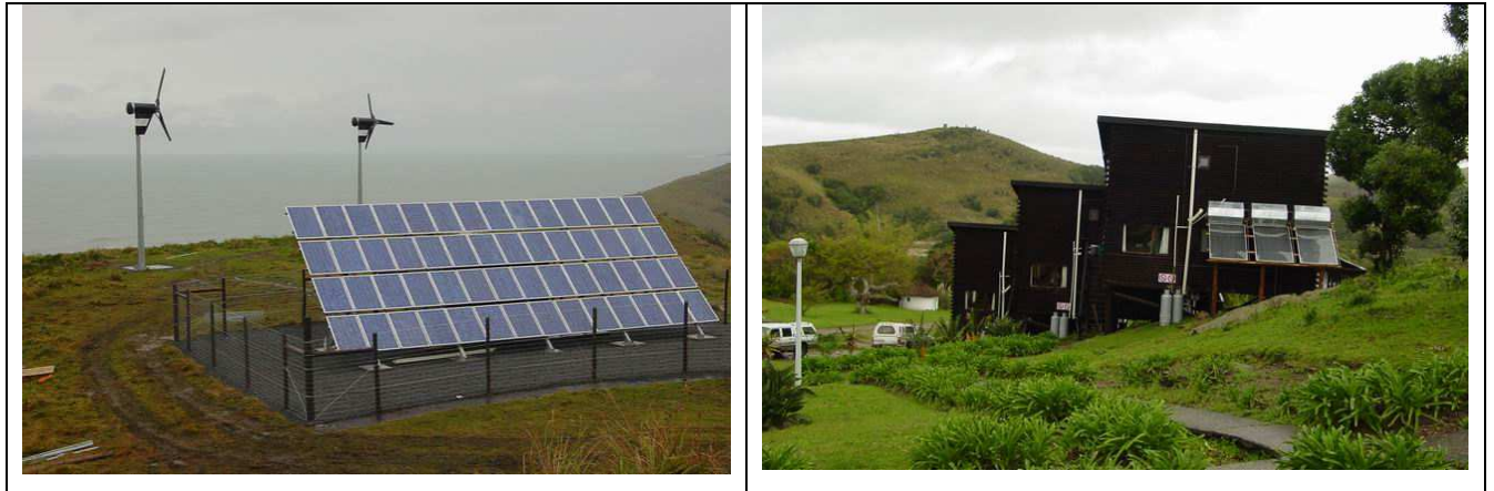
Figure 7: Solar water heaters and LPG bottles installed in Hluleka Nature Reserve
