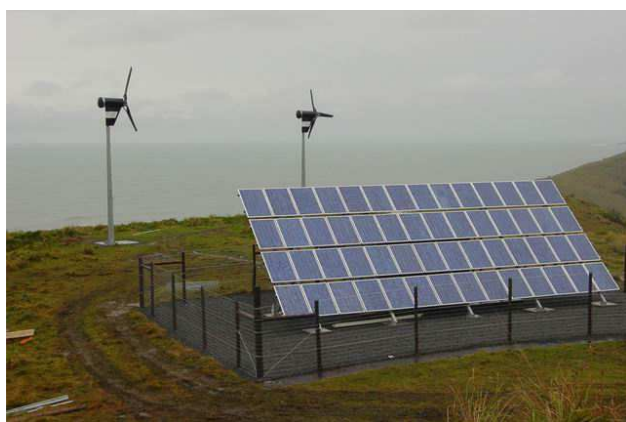
Figure 7. Wind, PV array at Hluleka Nature Reserve
