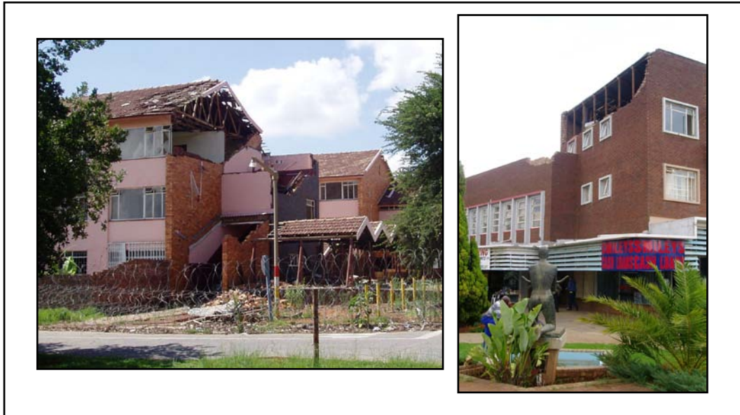
Figure 21. Damage to buildings in Stilfontein following a magnitude 5.3 mining-related earthquake (from Durrheim et al. , 2007)
