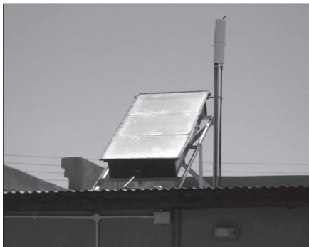
Figure 7: Solar geyser installed in a Hull Street Source: Matsebe, 2008
