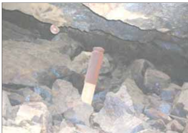
Figure 19—Down-dip edge of the pillar, showing the hangingwall blocks that fell out as a result of time dependant hangingwall deterioration adjacent to the pillar
