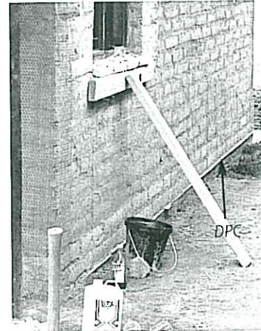
A damp-proof course has been put in the wall of this house
