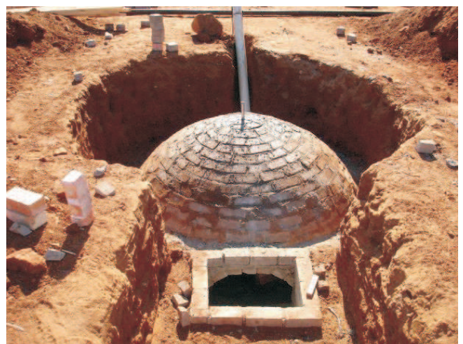
Fig. 1: The construction of a digester in Mpumalanga, South Africa (Picture: Jotte van Ierland).
