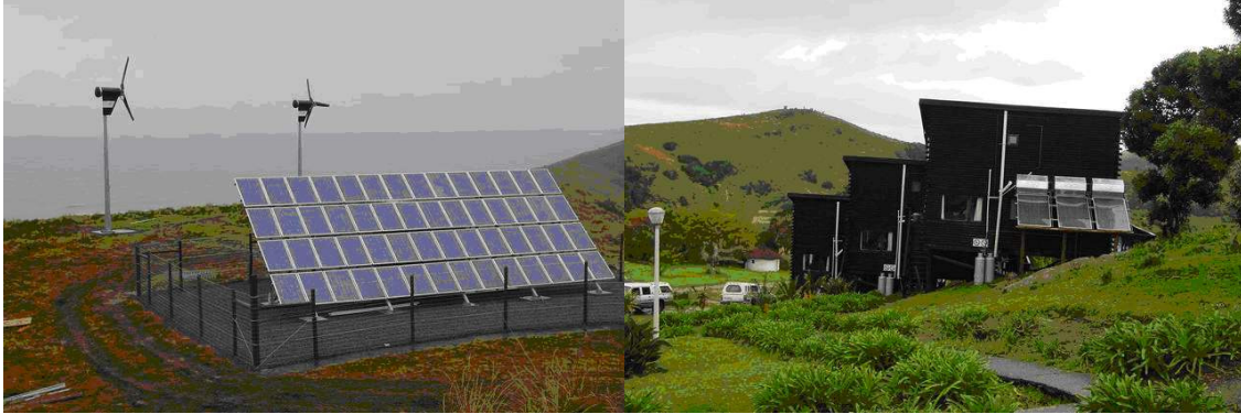
Fig. 1:: Wind, PV array and solar water heaters and LPG bottles at Hluleka Nature Reserve
