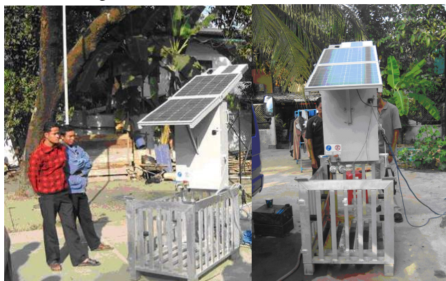
Fig. 5: Field test of a off-grid WaterPPS in Laos, Since January 07.
