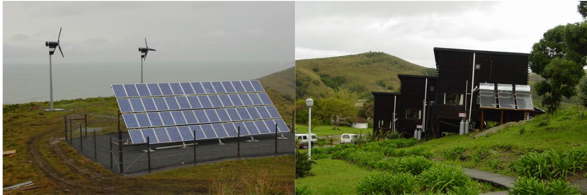
Figure 4: Wind, PV array and solar water heaters and LPG bottles at Hluleka Nature Reserve
