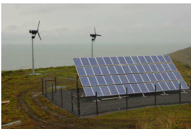
Figure 4: Wind, PV array at Hluleka
