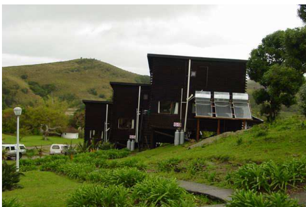
Figure 5: Solar water heaters and LPG bottles
