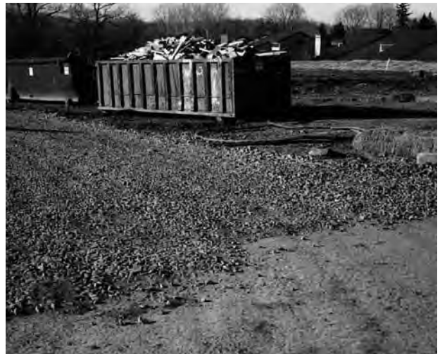
Figure 6.26 (a): Construction sites can be prevented from polluting the surrounding area by the use of straw bales, mulching and geo-mats. Aggregates placed at exits from sites prevent the transport of pollution
