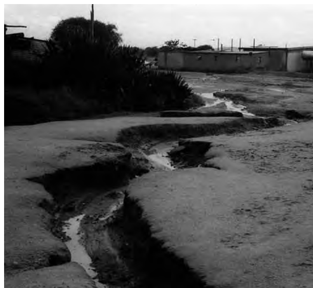
Figure 6.18 (b): Concentration of stormwater drainage in a roadway resulting in major inconvenience to road users
