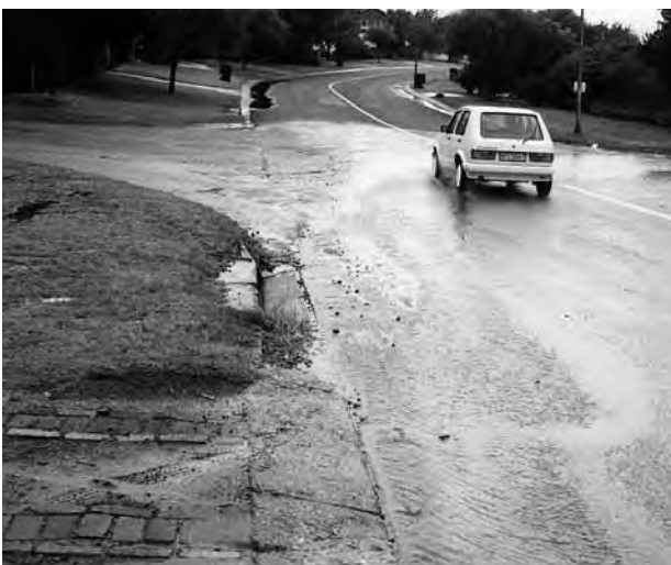
Figure 6.12: Incorrect vertical alignment has caused stormwater to bypass this kerb inlet. Kerb inlets in the intersecting road on the left have also not captured runoff from that road so that stormwater flows across this bus route, creating a hazard
