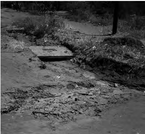
Figure 6.35: The use of underground drainage systems in unpaved roadways should be justified
