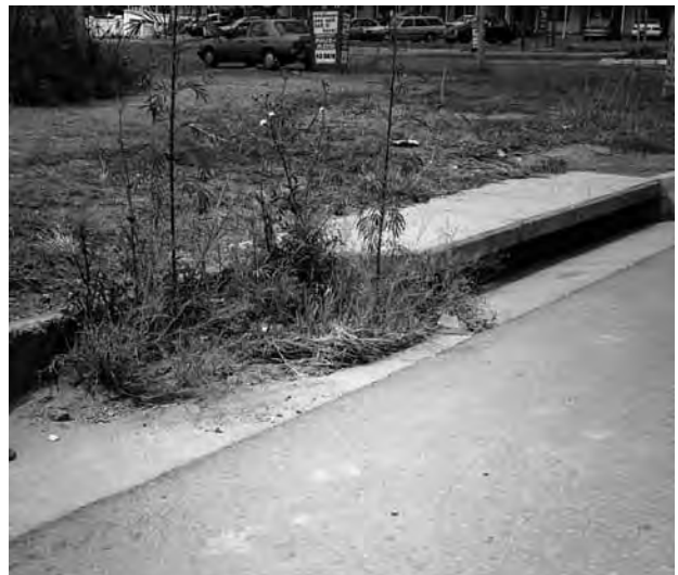
Figure 6.34: Kerb inlets require maintenance
