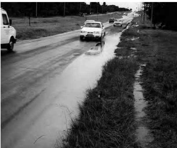
Figure 6.13: This ponding is the result of encroachment of the grass verge onto the road. Grass-cutting maintenance operations should also include harvesting the grass, to prevent siltation and build-up of new grass growth
