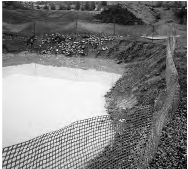
Figure 6.26 (b): Construction sites can be prevented from polluting the surrounding area by the use of straw bales, mulching and geo-mats. Aggregates placed at exits from sites prevent the transport of pollution
