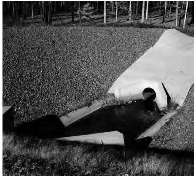
Figure 6.7: Multiple-outlet structure of a detention pond
