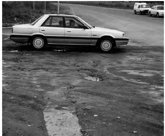
Figure 6.14: Flow across this intersection has resulted in siltation, which is inconvenient and hazardous to road users
