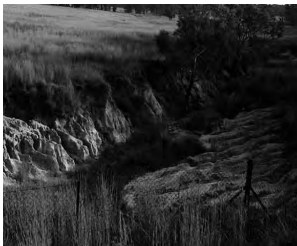
Figure 6.23: Gully erosion by headwater upstream of a highway culvert inlet. Specific attention needs to be paid to structures founded in soils with high erosion potential
