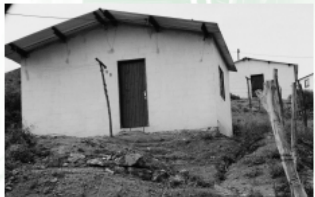
Fig. 1: Soil erosion in new housing development, Moirivier, South Africa.
