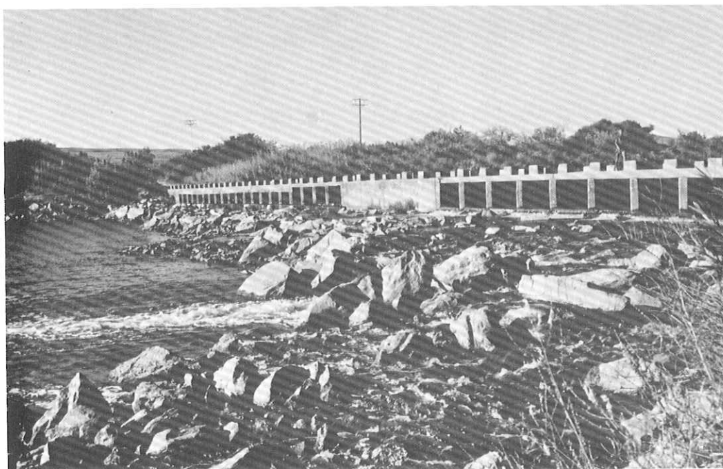
Fig. 5 : The "low water" bridge at Lutzville which marks the head of tidal effect in the Olifants River some 32 km from the sea (measured along the river course).
