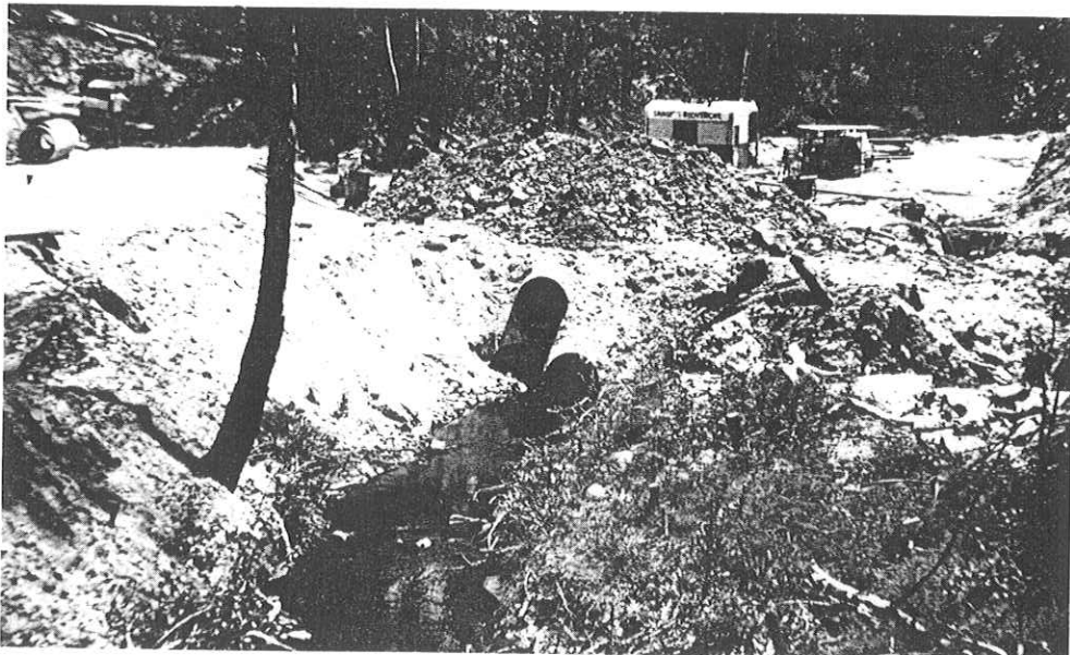
FIG. 5: The new Onrus/Hermanus highway bridge under construction. Temporary gravel fill threatens to add further sediment to the Onrus Lagoon unless there is thorough rehabilitation after completion of the bridge (ECRU 79-12-06).
