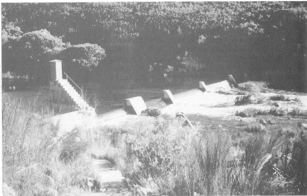
FIG. 11: The gauging weir (Welgemoed) just above the coastal road bridge. (Photo: ECRU, 86-08-20).
