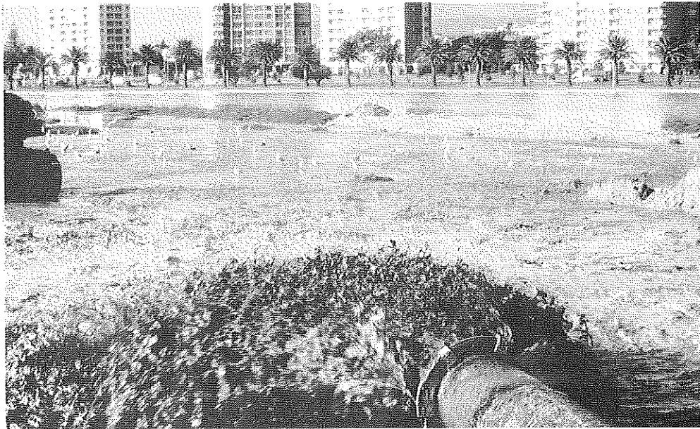
FIG. 11: The foundation for the development of the Woodbridge Island Development depended upon sandfill pumped from the bed of the lagoon by a dredger. (Photo: J R Grindley).
