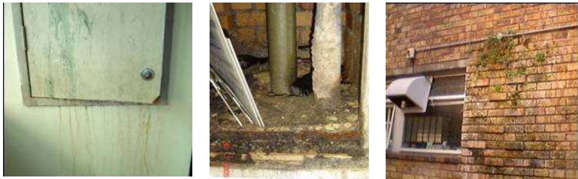
Figure 3: Duct to Service Duct, Inside Service Duct and External Wall outside Service Duct
