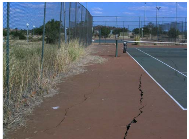
Fig 9. Damage to tennis court – note distortion of fencing supports
