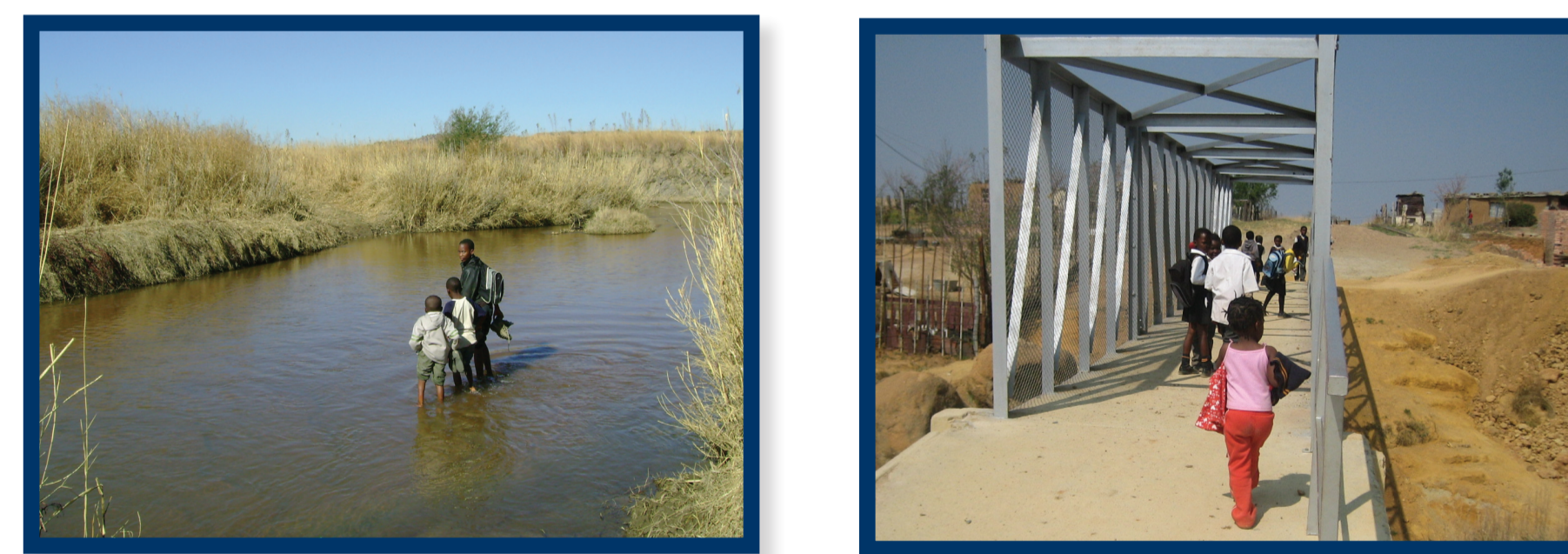
Before intervention (left): Learners wading through water in the Mpuluzi River. After intervention (right): Learners walking across the newly-constructed pedestrian bridge across the Mpuluzi River
