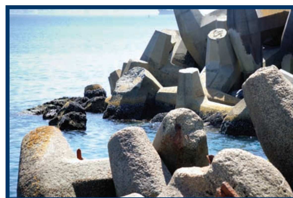
Figure 2: Close-up of dolosse, showing damage and wear.
