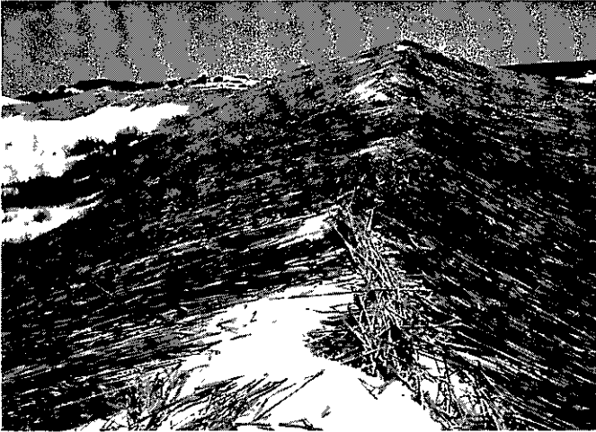
PLATE 130. Method of laying reed mats perpendicular to the slope and meeting along crestlines. Elands Bay.
