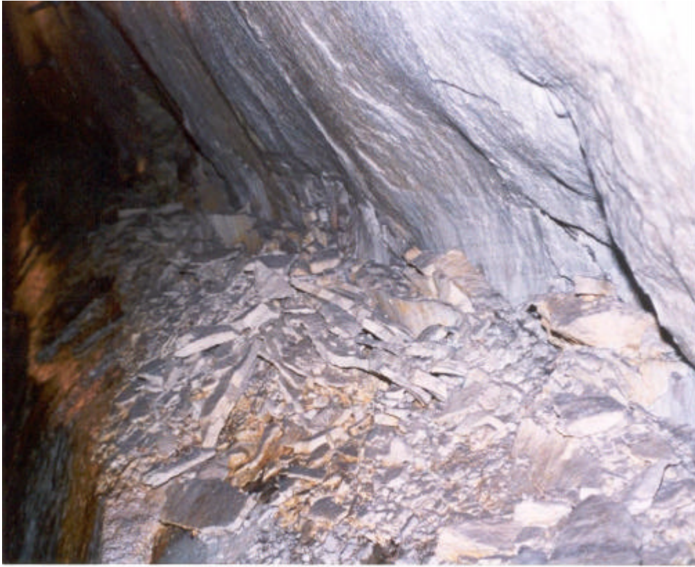
Figure 11 Dog earring in a 5m diameter tunnel
