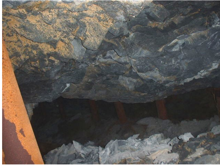
Figure 4.3.8 Fall of ground at the bottom of E8.
