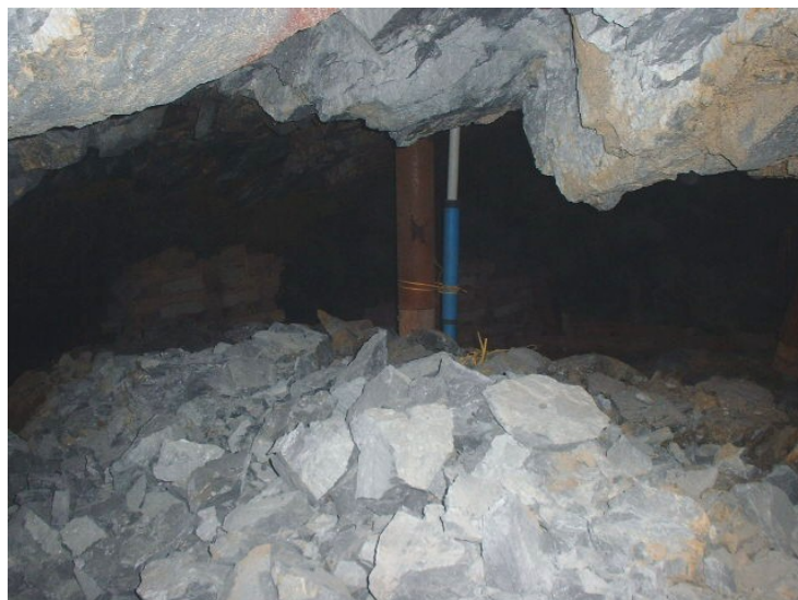
Figure 4.3.7 Fallouts around the 0311 closure meter in panel E10.
