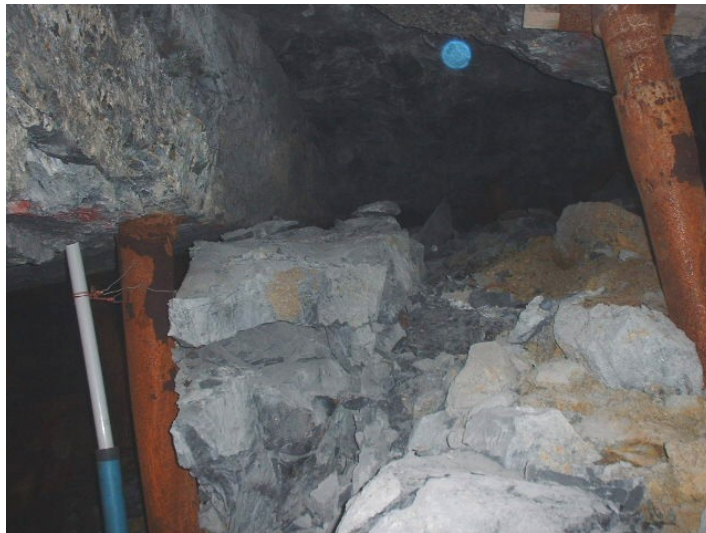
Figure 4.3.4 A different view of the fallout in Figure 4.3.3 to illustrate the fallout height.
