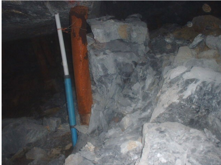
Figure 4.3.3 Fall of ground in the E10 panel next to the 0249 closure meter. The fallout height was approximately 1 m.
