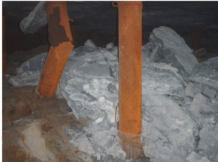
Figure 4.3.6 Fall of ground in the back area of E10.
