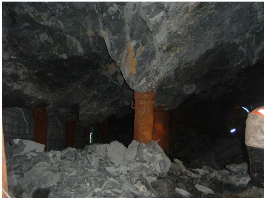
Figure 4.2.6 Fall of ground in the E8 panel showing the zone of influence of the support unit.
