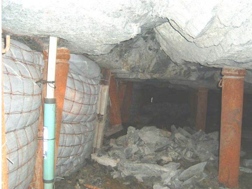
Figure 4.2.3 Fall of ground in the E8 panel next to the 0306 closure meter (looking down dip).
