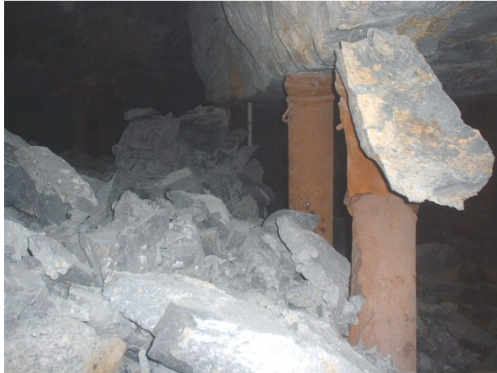
Figure 4.3.5 Fall of ground in the back area of E10.
