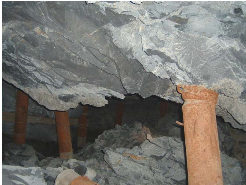
Figure 4.2.5 Fall of ground in the E8 panel close to the bottom gully.
