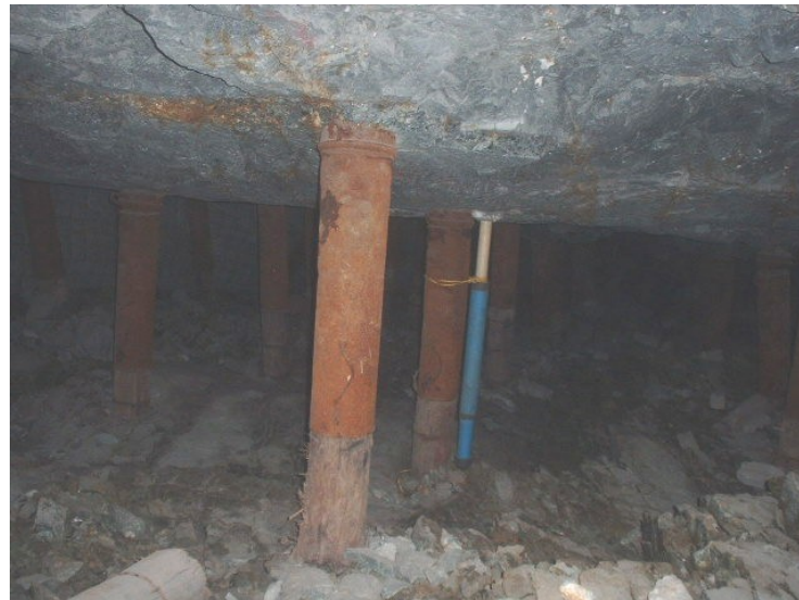
Figure 4.3.9 Hangingwall conditions in the E7 panel after the seismic events showing very little damage.
