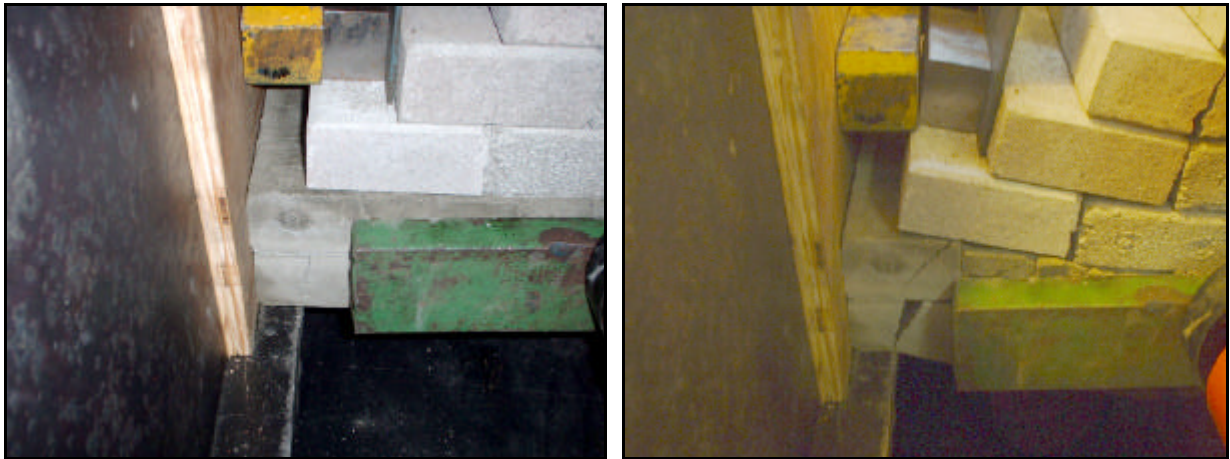
Figure 32. Progression of cracks in concrete blocks
