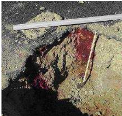
Figure 3 - The stabilised layer shows no signs of the carbonation reaction, note how dry the surfacing is (Semmelink et al, 2002)
