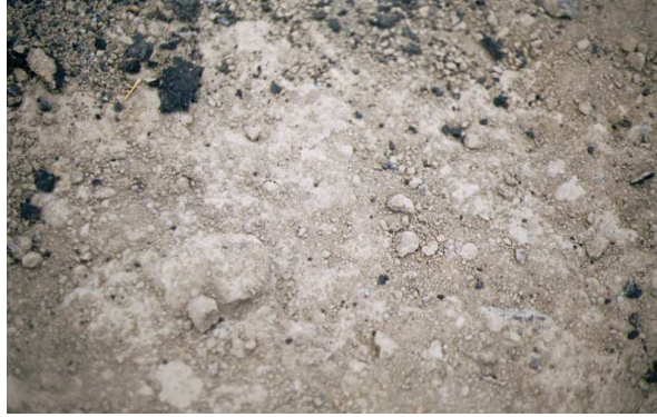
Figure 4 - Close-up view of surface of recycled weathered dolerite surface where the surfacing broke loose showing the loose material
