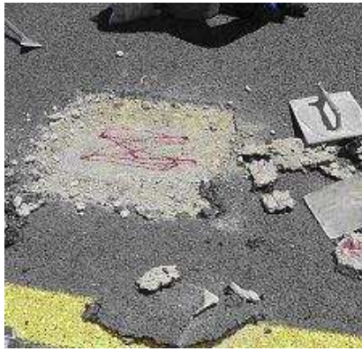
Figure 2 - The dry layer under the Bitumen-Rubber seal is shown in the photograph, limited CO 2 exposure and a built up of moisture under the seal has created this condition. The carbonation tests show that no carbonation took place, the dry condition shows the destructed top portion of the layer (Semmelink et al, 2002)
