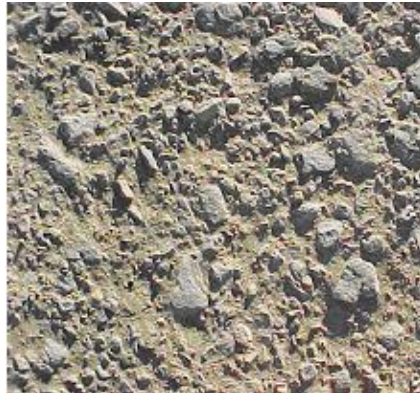
Figure 1 - View of the broomed surface of stabilised base showing coarse finish after removal of fines which did not stabilise and compact just before priming and sealing, shortly after stabilisation before priming and surfacing (taken at the time of construction)(Simmelink et al, 2001)
