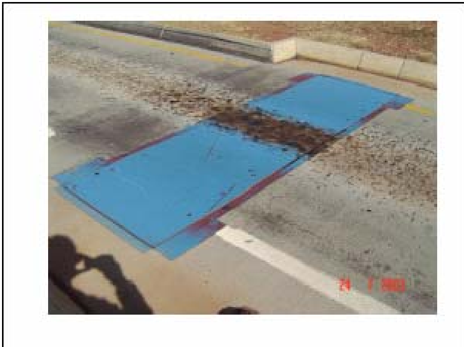
Figure 2: DAW 50 in position (permanent installation) at the N3-TCC (in front of the SIM system)
