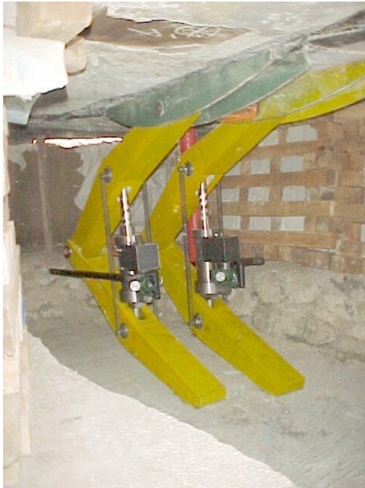
Figure 5-6: Photo of roof support system in training mock-up stope of Kloof mine.
