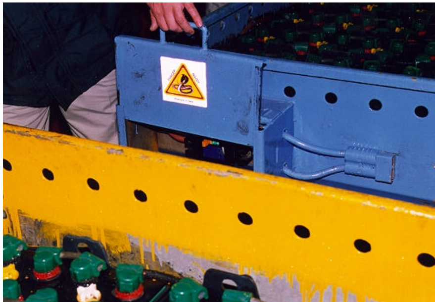
Figure 4.2.5.3: Isolating switch location
