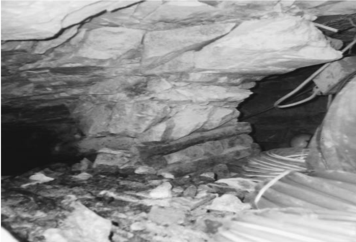
Figure 1.1 The zone of influence of a mat pack after a seismic event (courtesy Hartebeestfontein Gold Mine)
