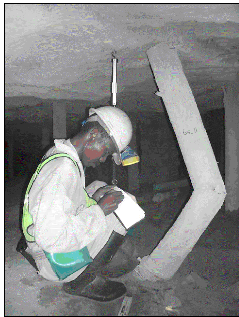
Figure 4.5.2 Photograph showing the buckling failure mode.
