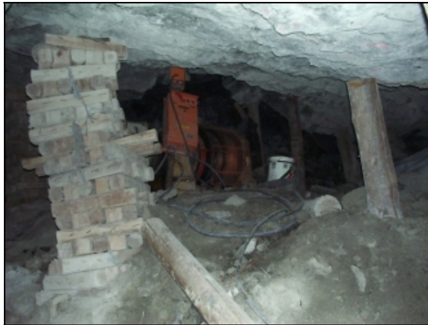
Figure 2.3.9 Photograph showing the rotation of support elements during a collapse.
