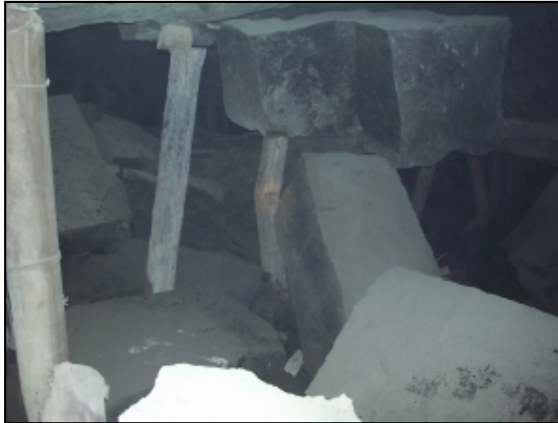
Figure 2.3.8 Photograph showing cantilever-type block rotation.
