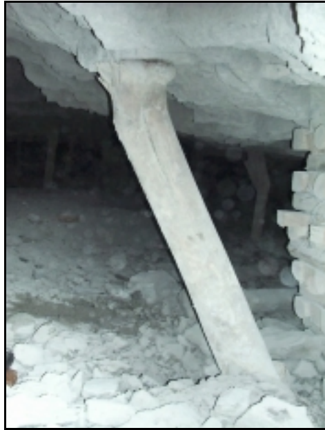
Figure 4.5.3 Photograph showing the brushing failure mode.
