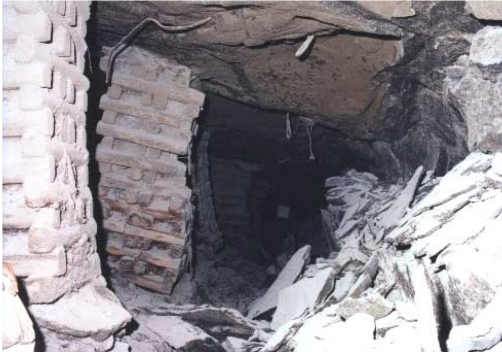
Figure 4.20 - Merensky Reef - no siding. Severe spalling down-dip
