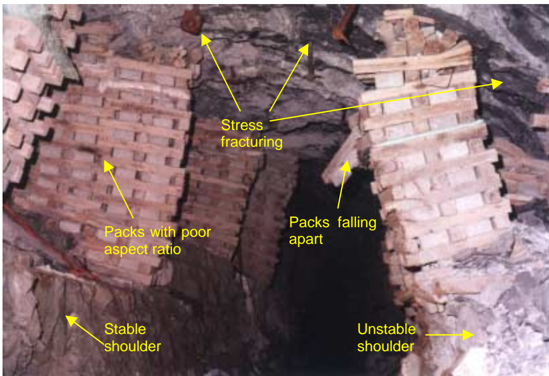
Figure 4.33 – VCR - Typical conditions that may develop along a gully created as an ASG with lagging siding under high stress
