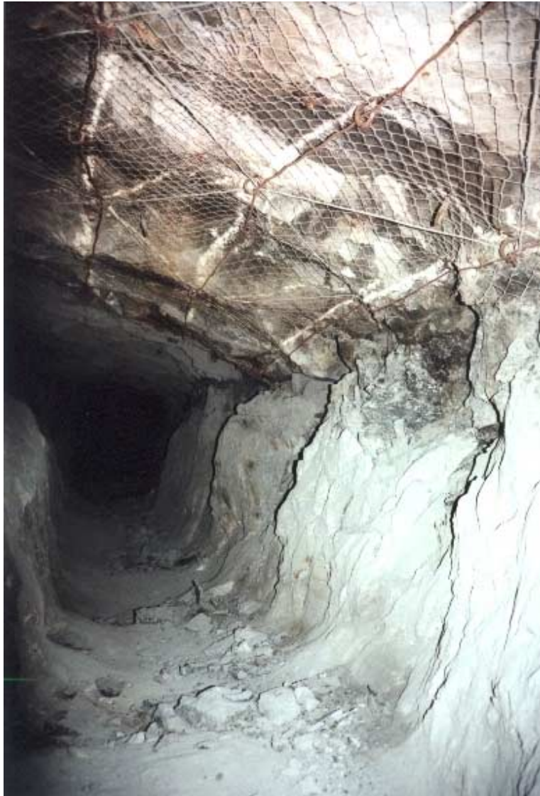
Figure 4.19 - Merensky Reef gully where a crush pillar lies on the gully edge and during crushing has damaged the hangingwall resulting in mesh and lacing application to control minor falls
