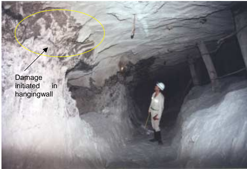
Figure 4.15 - Gully with no siding on the Merensky Reef at 800 m depth. Conditions are stable, although spalling has clearly occurred along the pillar sides. Note that pillar edge damage runs up and into the hangingwall.
