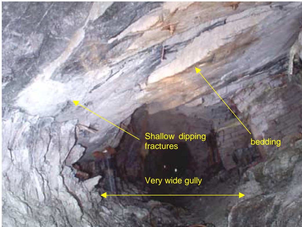
Figure 4.27 - Basal Reef – the effect of a lagging siding on hangingwall conditions – view from face area looking back along gully
