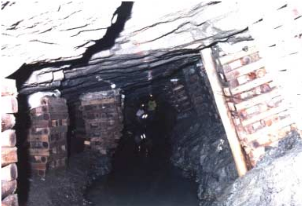
Figure 4.21 - Gully with lagging siding. Down-dip siding has a flat floor due to stress fracture damage. Down-dip packs are vertical
