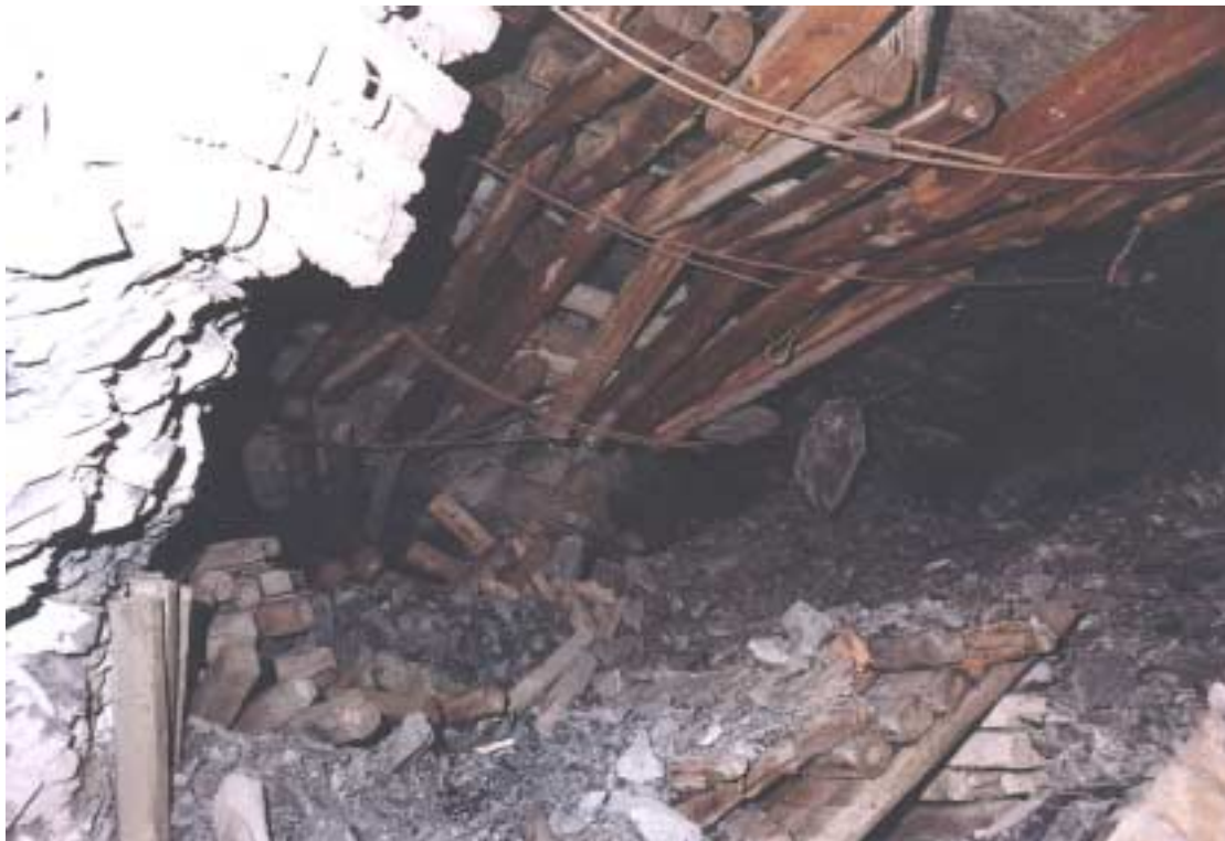
Figure 4.39 – Roadway after seismic damage – packs collapsed, trusses and hangingwall intact (after rockburst)
