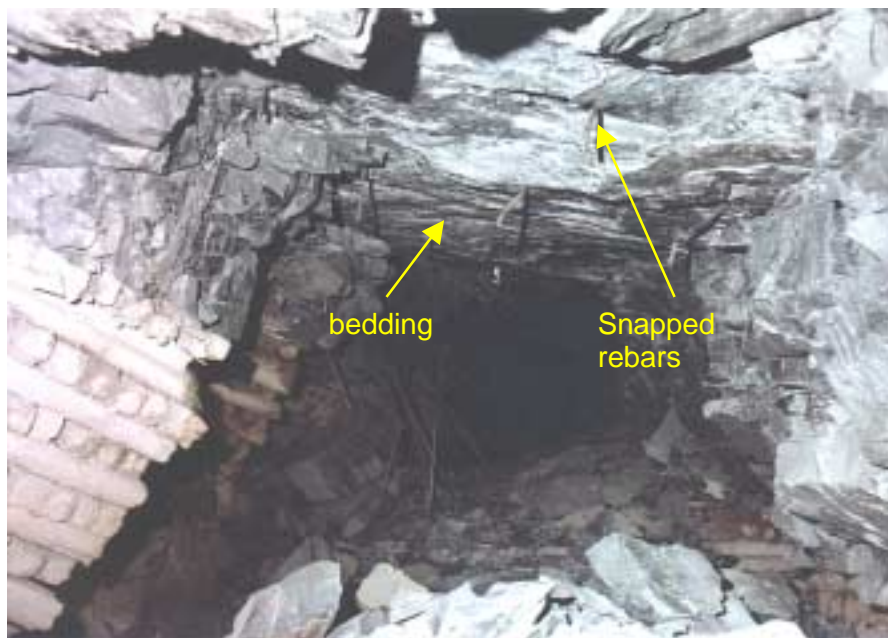
Figure 4.36 - Collapse back along a gully as a result of seismic activity. The hangingwall has collapsed between packs up to a bedding parting. Rebars are snapped or exposed
