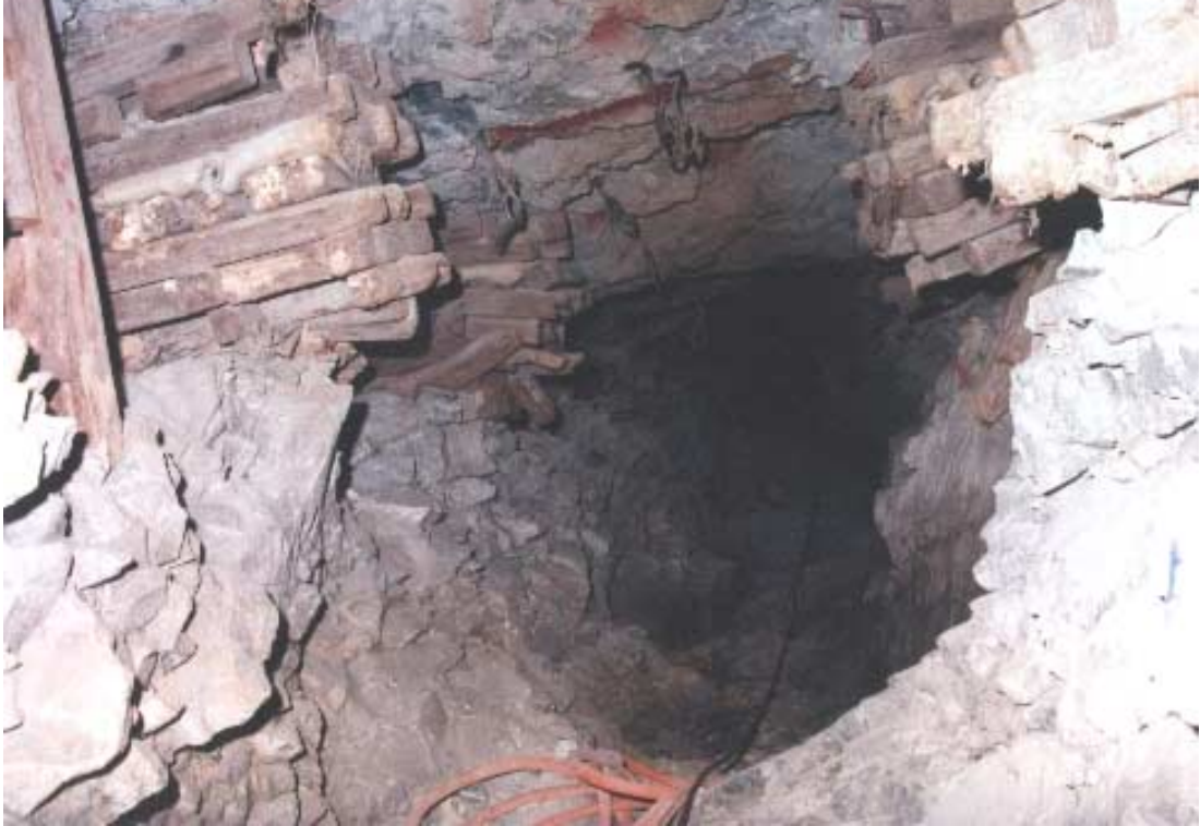
Figure 4.45 – VCR - Poor footwall lifted gully conditions resulting from blasting practice where holes are drilled downward into the stope footwall and a long distance of gully is ripped simultaneously.
